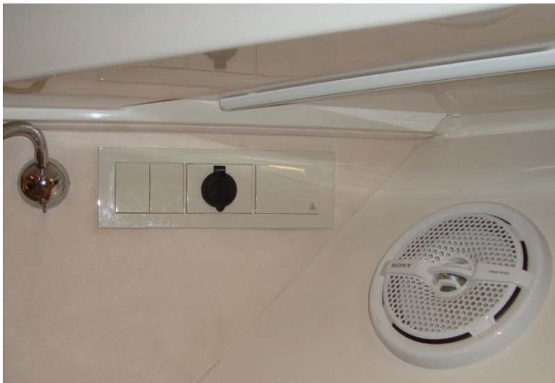
Picture 44: 230V socket in the front cabin.
