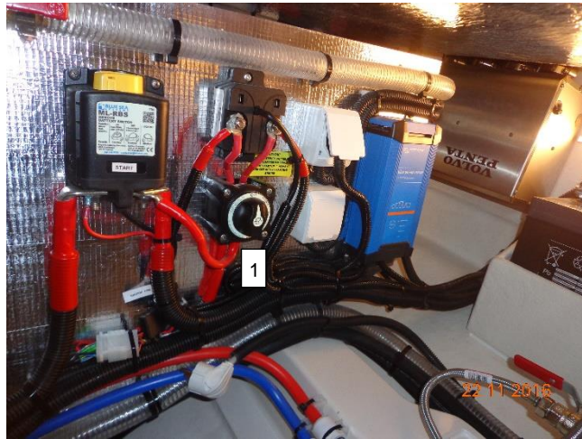
Picture 37: Batteries crossover switch (1).
