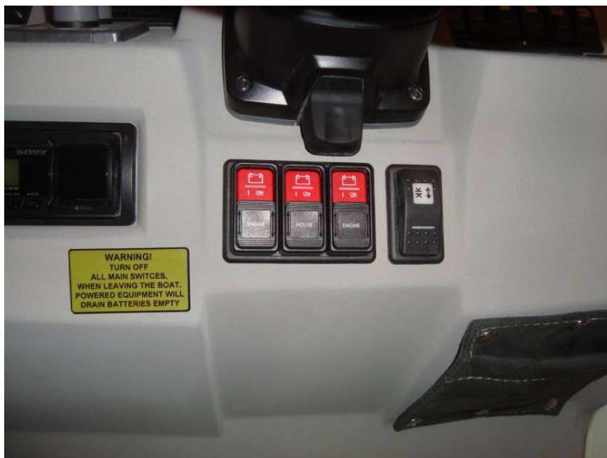
Picture 39: Main switch panel
