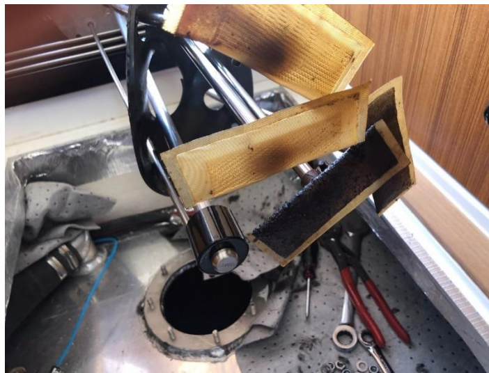
Picture 58: Fuel filters in fuel tank.
