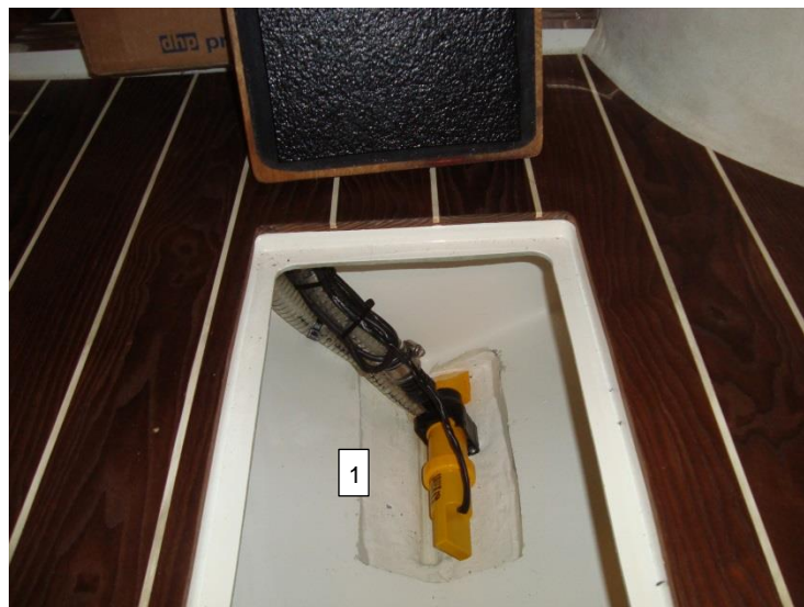
Picture 60: Pump inlet in the front cabin area (1)
