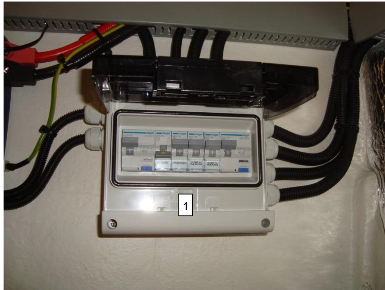
Picture 30: 230 V Main fuse 20A and grounding relay (1) (Lamp indicates when 230 V is active.)
