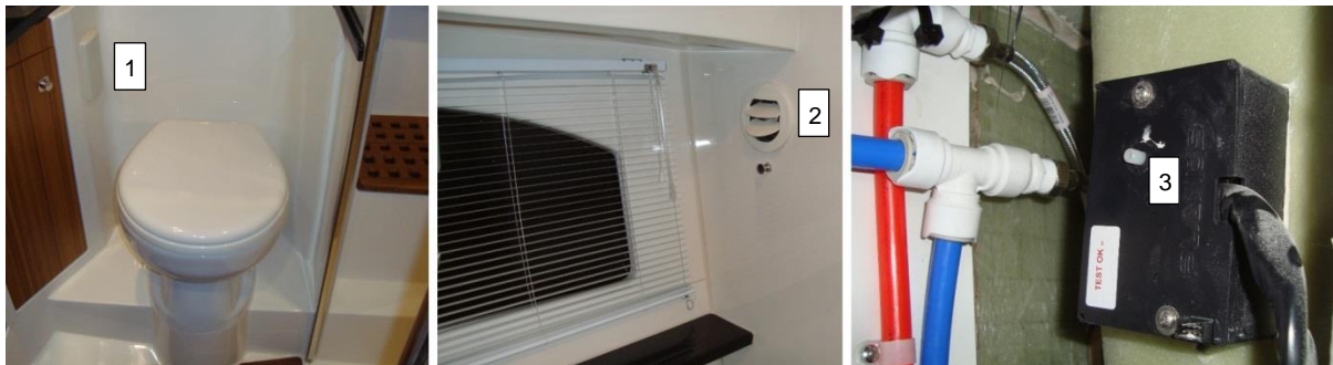
Picture 24: Toilet controls (1), ventilation (2), water level trimmer shaft (3)
