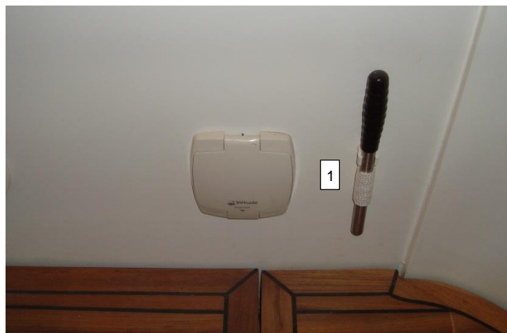
Picture 17: Manual bilge pump for the engine room (1)
