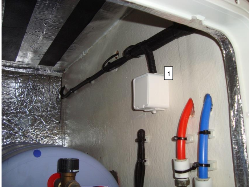
Picture 41: 230V socket on port side in the engine room, charger (1).
