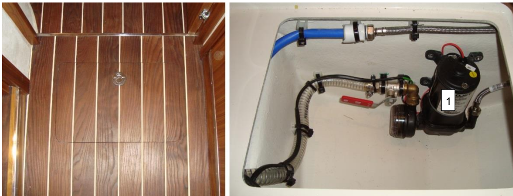
Picture 21: Fresh water pump and filter under the hallway floor (1)
