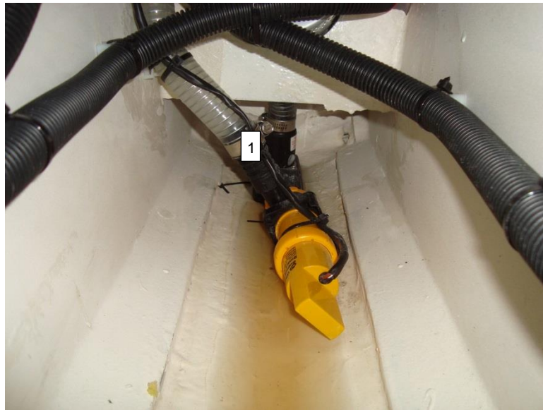
Picture 59: Pump inlet in the engine room (1)
