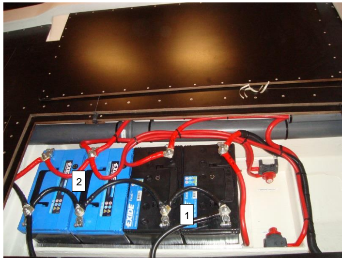
Picture 27: Starter batteries (1) Service batteries (2)
