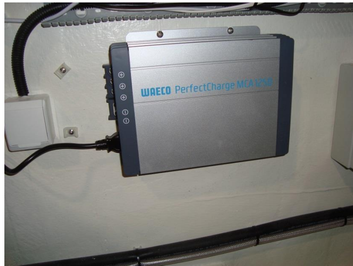
Picture 29: Dual sense charging relay
