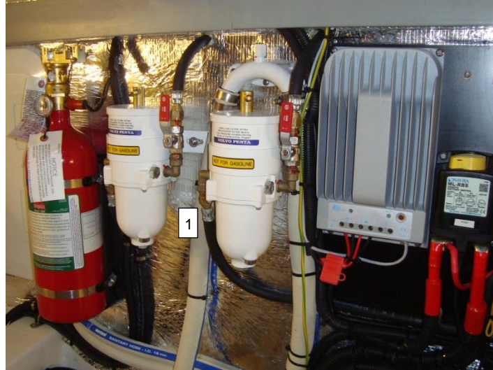
Picture 14: Two diesel filters with water separators (1)
