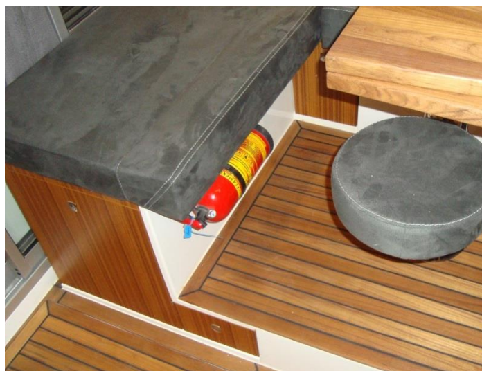
Picture 33: Portable fire extinguisher - 2 kg capacity (1)
