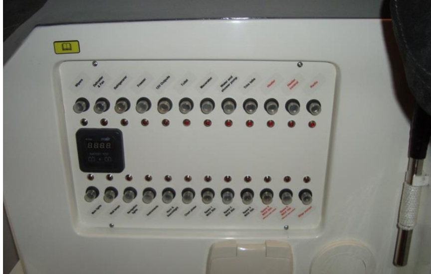
Picture 38: The fuse panel
