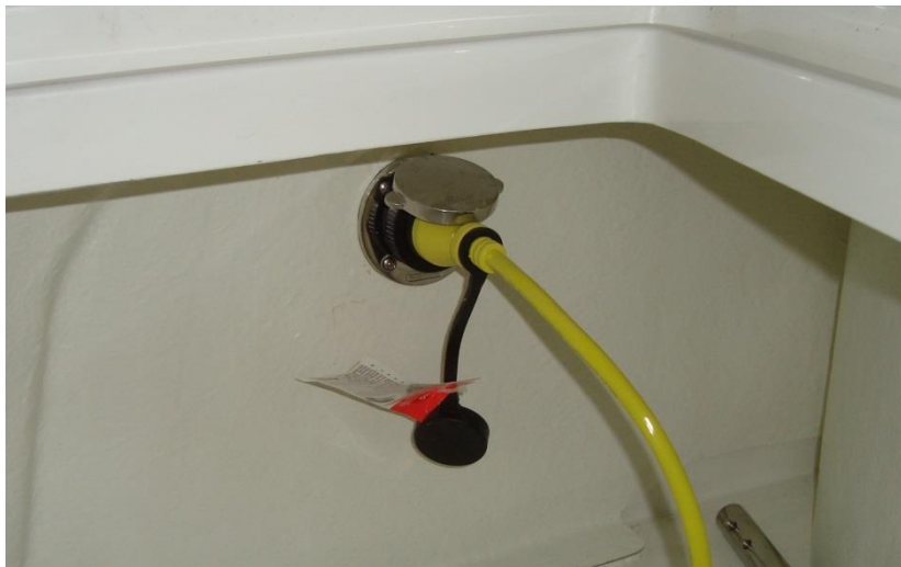
Picture 47: The shore connection.
