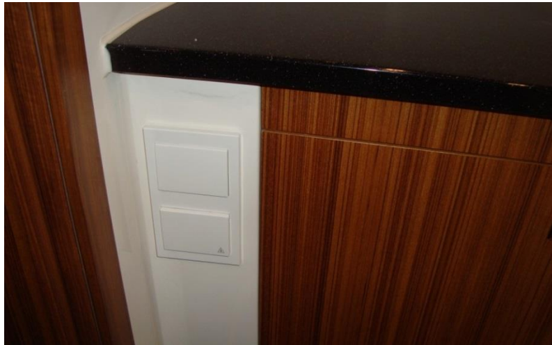
Picture 43: 230V socket in the toilet room.
