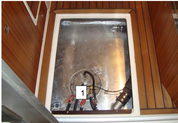
Picture 9: 2 Emergency fuel closing valves – cockpit (1)
